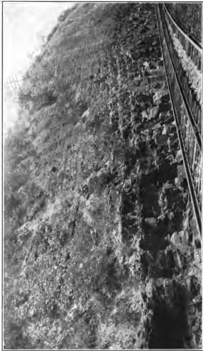
PLATE XV. —Anticline in Hamilton Shales (West End) with Heavy Sandstone Stratum at Base, in deep cut of Baltimore and Ohio Railroad North of North Mountain Station.
